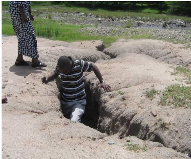
Plate 2: Gully erosion in Malekano village Simiyu river catchment. Source: GoT, 2012
